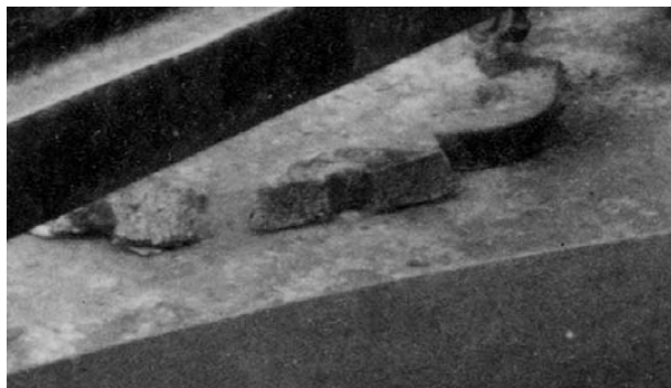
13 Closeup of three broken lugs from twelfth pier. The centre sample shows numerous crack arrest lines with a small blowhole on the lefthand wing of the lug, probably indicating intermittent crack growth (fatigue)
